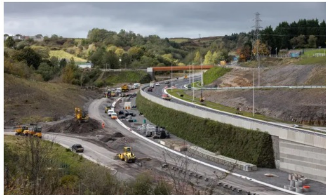
Work on the construction of a dual carriageway between Brynmawr and Gilwern in Wales. Projects that are in progress are expected to continue as planned. Photograph: Huw Fairclough/Getty
